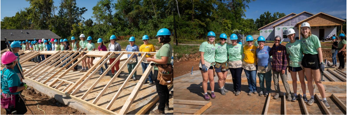
Photo on the right: St. Thomas builders Lydia Arnold, Kim Arnold, Gretchen Moehlmann, Pr. Adrienne, Pr. Lecia, Mary Moore, Eve Arnold, and Rebekkah Arnold on the build site.
